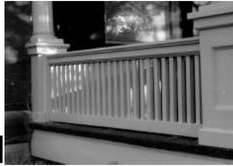
When replacing missing porch railings, the proportions and spacing of balusters should match the original. This replacement matches the original.
