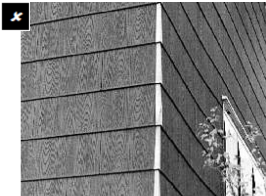
Imitation materials that are designed to look like wood or masonry siding, but that are fabricated from other materials, are inappropriate.
