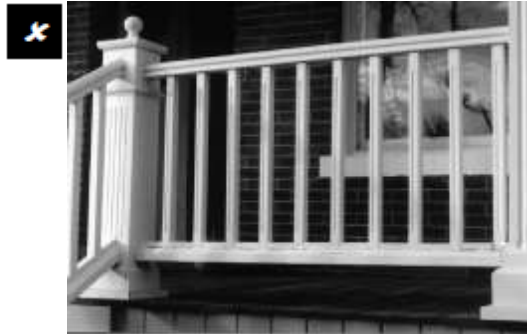
The spacing of balusters on this replacement railing is inaccurate.
