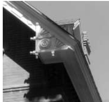
Features such as eave details often exhibit materials and finishes associated with particular styles, and therefore their preservation is important.
