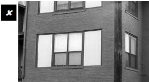
Enclosing a historic window opening on a key character-defining facade destroys much of the building's historic character and is inappropriate.
